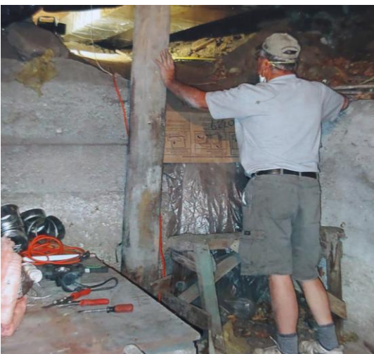
Hal Becker assessing the damage.
